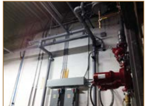
Figure 10, Pumps and Valves
