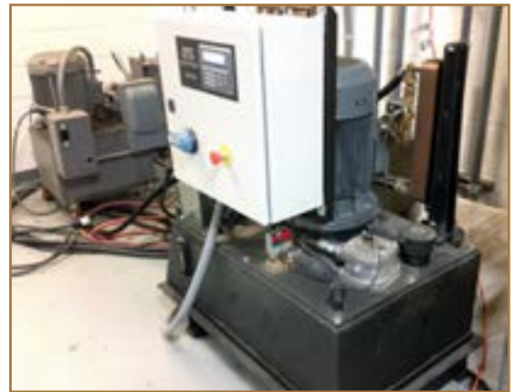
Figure 2, Hydraulic Power Units
