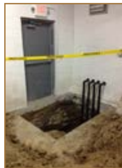
Figure 4, Geothermal Pipes Enter the Building
